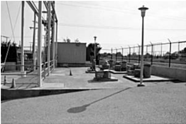
Matadero Storm Water Pump Station
